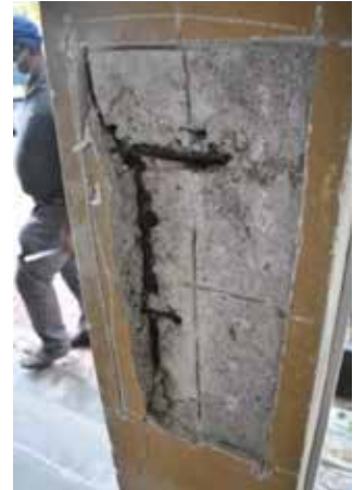
Figure 3: Corroded G/F column School ID-N
