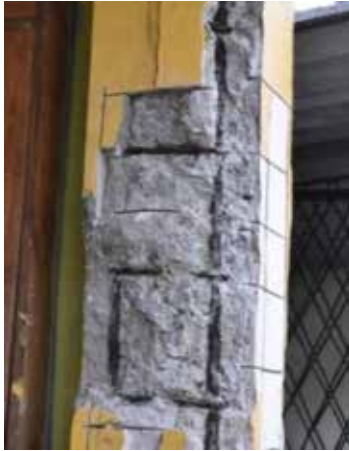
Figure 1: Corroded G/F column School ID-D
