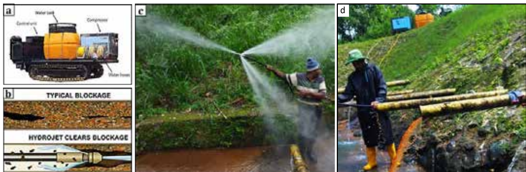
Figure 3: (a) The cleaning device, (b) Illustration showing the cleaning of blocked pipes using high-speed water, (c) High-speed water system used for cleaning at Watawala Landslide, (d) Hydro jet cleaning process of gravity drains in progress
