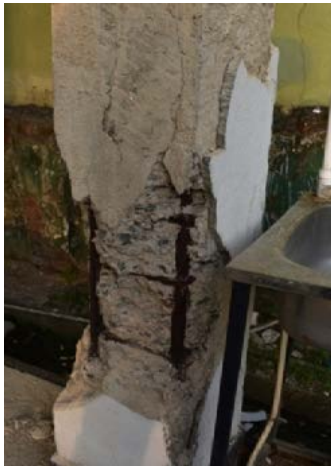
Figure 4: Corroded G/F column School ID-C
