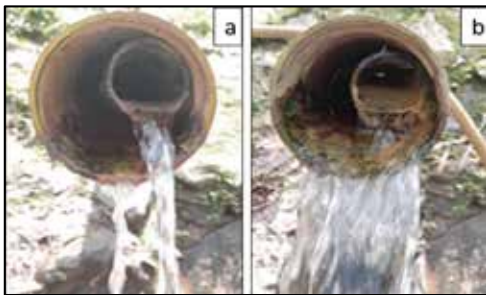
Figure 4: Photographs of the cleaning Directional gravity subsurface drain No. 10 a) before and b) after
