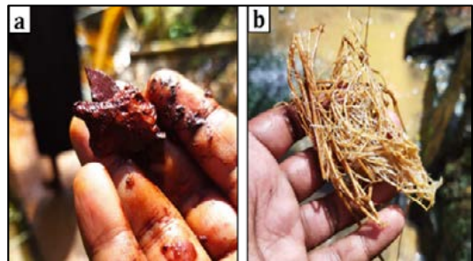
Figure 5: Obstructive materials encountered during the cleaning and flushing process using cleaning devices. a) Chemical and biochemical clogging with iron oxides b) Plant roots overgrowth inside the drain
