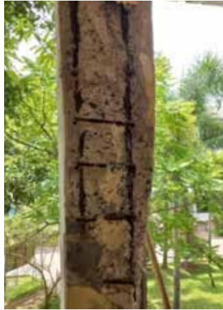
Figure 2: Corroded G/F column School ID-N
