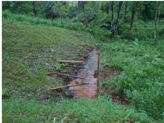
Figure 2: Directional gravity subsurface drains, which installed passing through the active landslide
