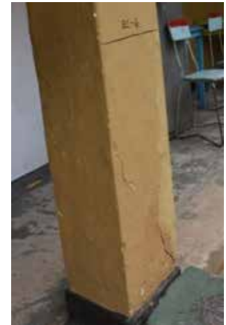
Figure 6: Fig .6.Cracked G/F column School ID-I2
