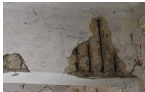
Figure 8: Corroded beam rebar, School ID-O
