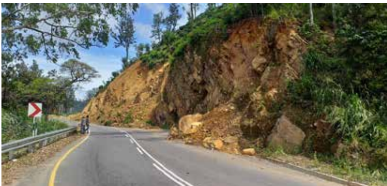
Figure 1: Road cut failure at Ch 140+560 of Peradeniya - Badulla - Chenkaladi Road (A5)
