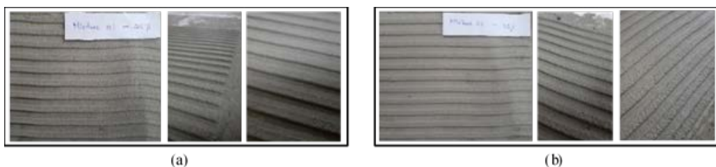
Figure 2: Cracking inspection results (a) M1 (b) M2
