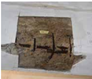
Figure 7: Corroded beam rebar, School ID-A
