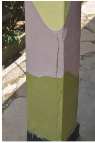
Figure 5: Cracked G/F column School ID-B
