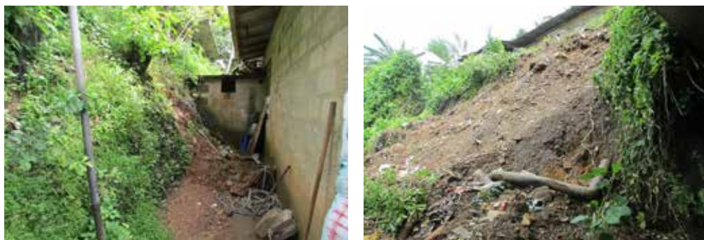
Figure 03: Photographs showing cut slope failures in the Bogahawaththa landfill
